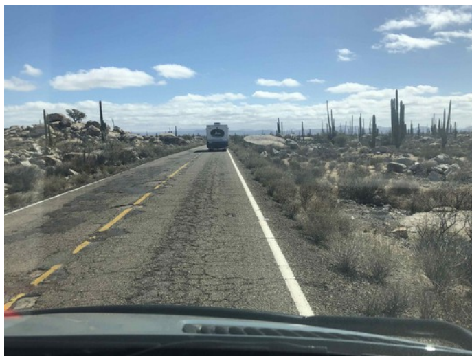
Of course, no trip to Mexico would be complete without mentioning the conditions of the highways and this stretch of Mex 1 between El Pabellon and Santa Ines was a tour guide's dilemma . We encountered frequent crater-sized pot holes, crumbling pavement, shoulders with sheer drop offs, and innumerable 18-wheelers traveling fast. Cautious driving was a must!
